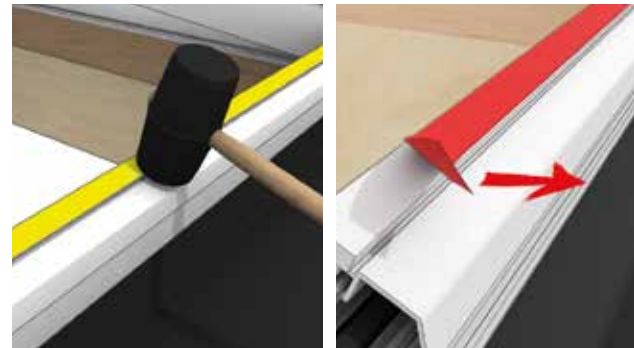
14 Clip trim onto the top of the ringbeam using a rubber hammer if required and then peel back the corner of the protective tape and fully remove.
